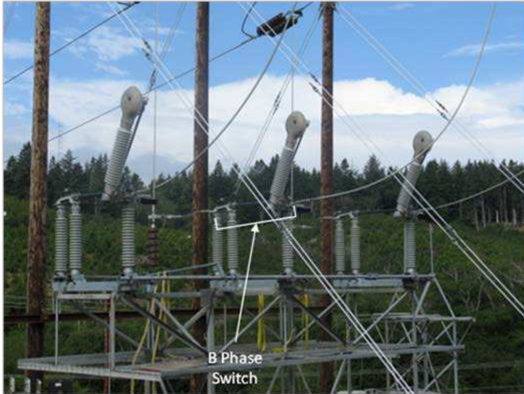
Figure 5: Structure 46/5S Switch B447
